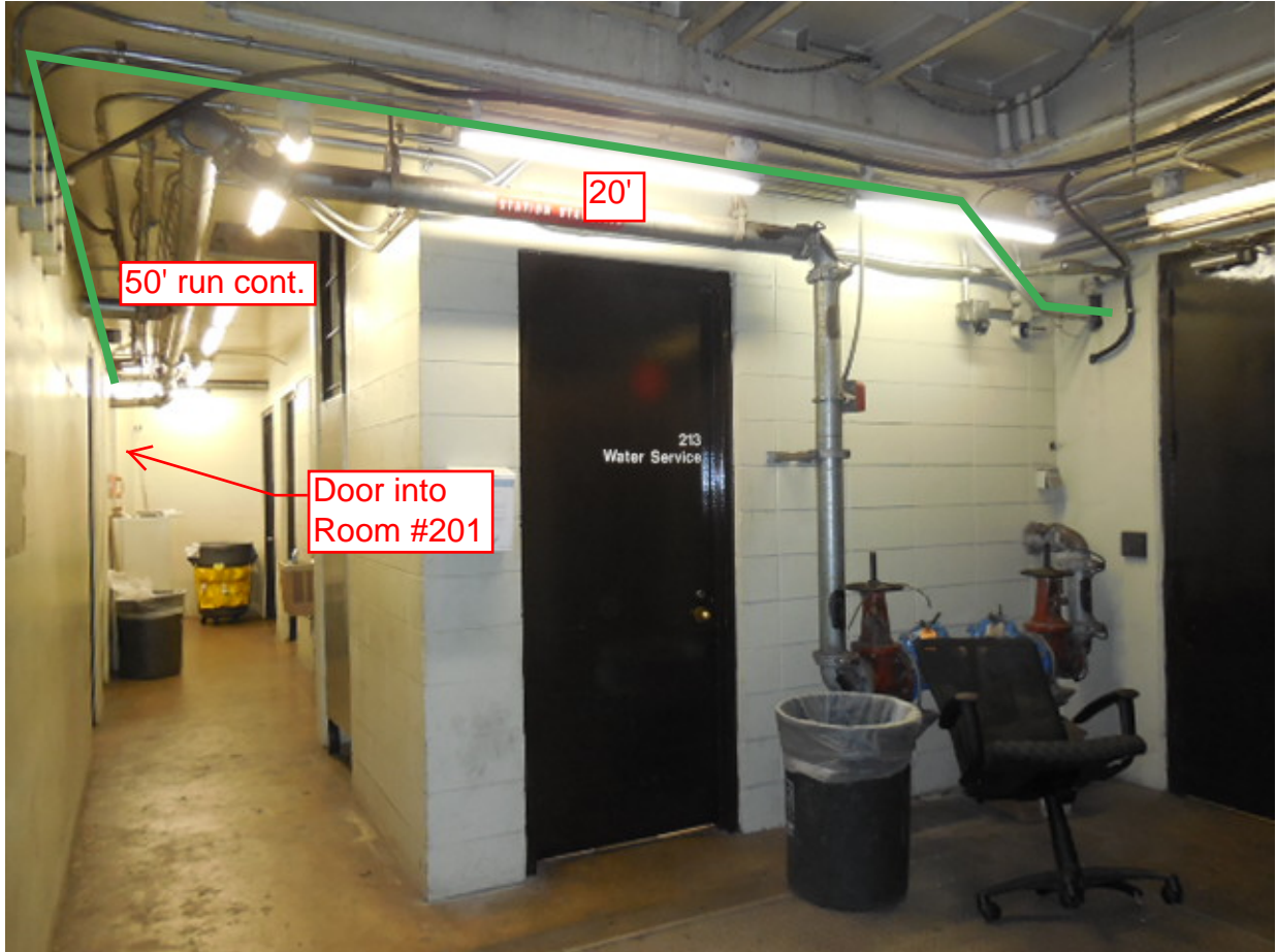
Photo #7 – A03 Dupont Circle South: Proposed conduit run continuing down hallway of room #201 and towards room #215
