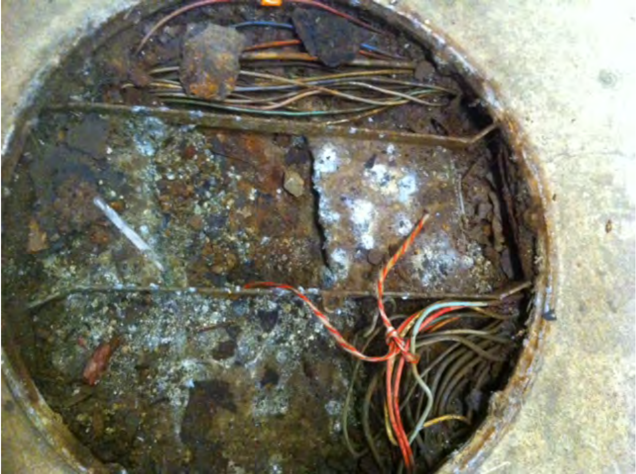
Photo #6: B07 Takoma – Poor conditions in second handhole
