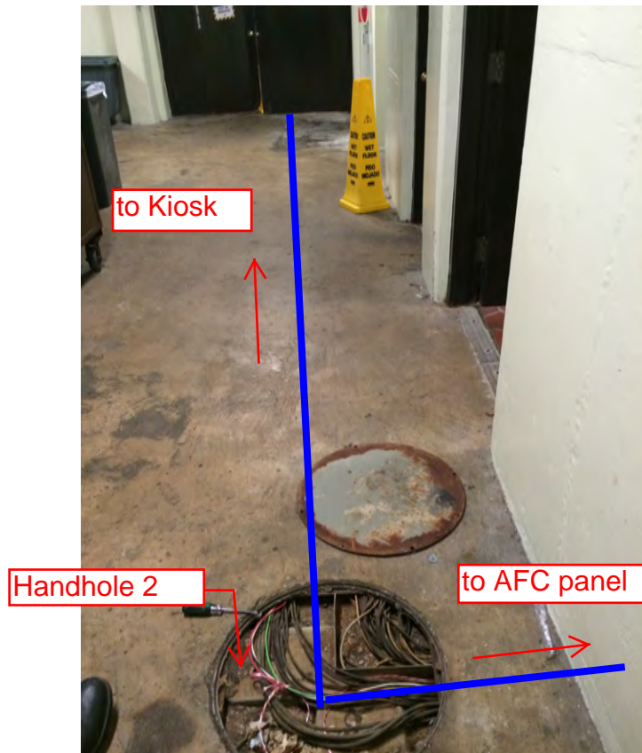
Rockville Photo #2 – Duct route between Kiosk and Electrical Room
