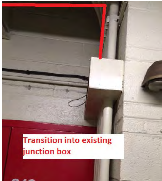
Farragut North NW Photo # 10 – Proposed conduit transition into existing junction box
