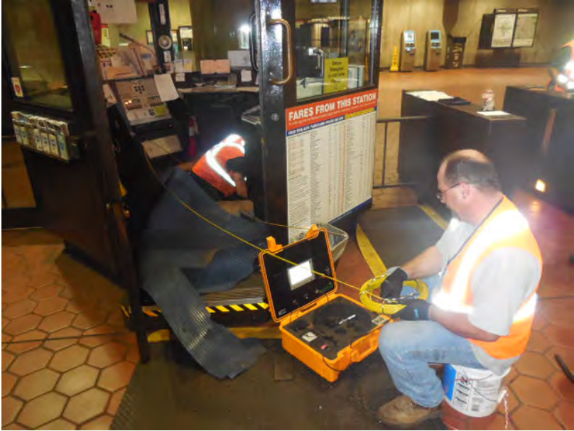
Photo #4: B10 Wheaton: Attempting to video-scope the faregate array ducts
