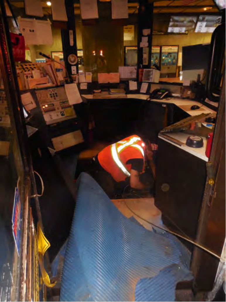
Photo #3: B10 Wheaton: Pushing in fish tape for the faregate array ducts
