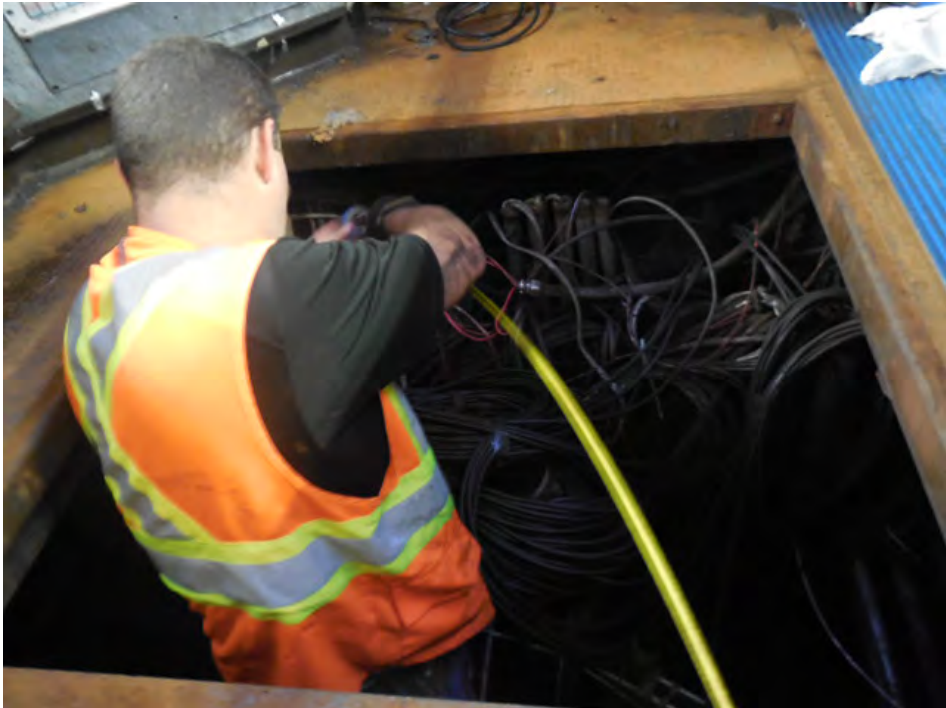
Photo #4: A08 Friendship Heights – Installing pull string between kiosk and AFC panel
