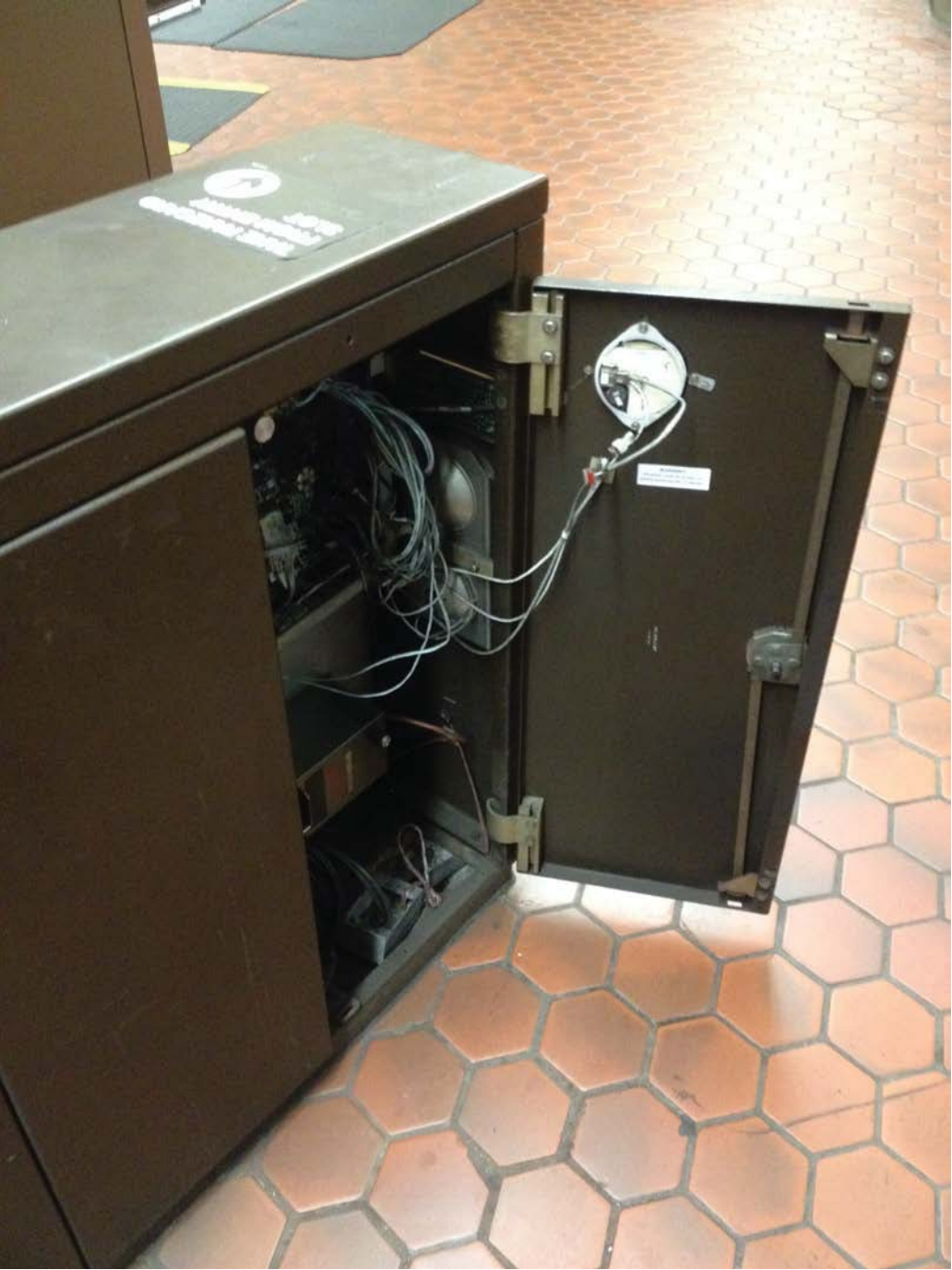
Photo #1: B02 Judiciary Square (East) – Faregate with new comm. duct and cable installed
