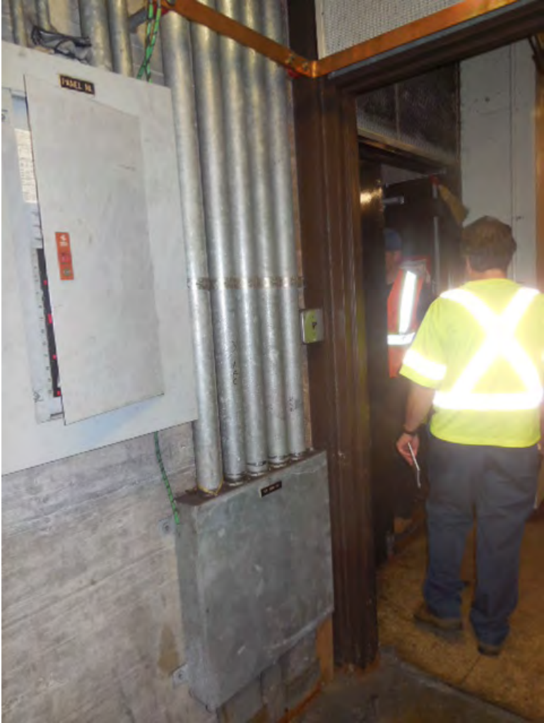
Photo #9: B10 Wheaton: Junction box near the AFC panel
