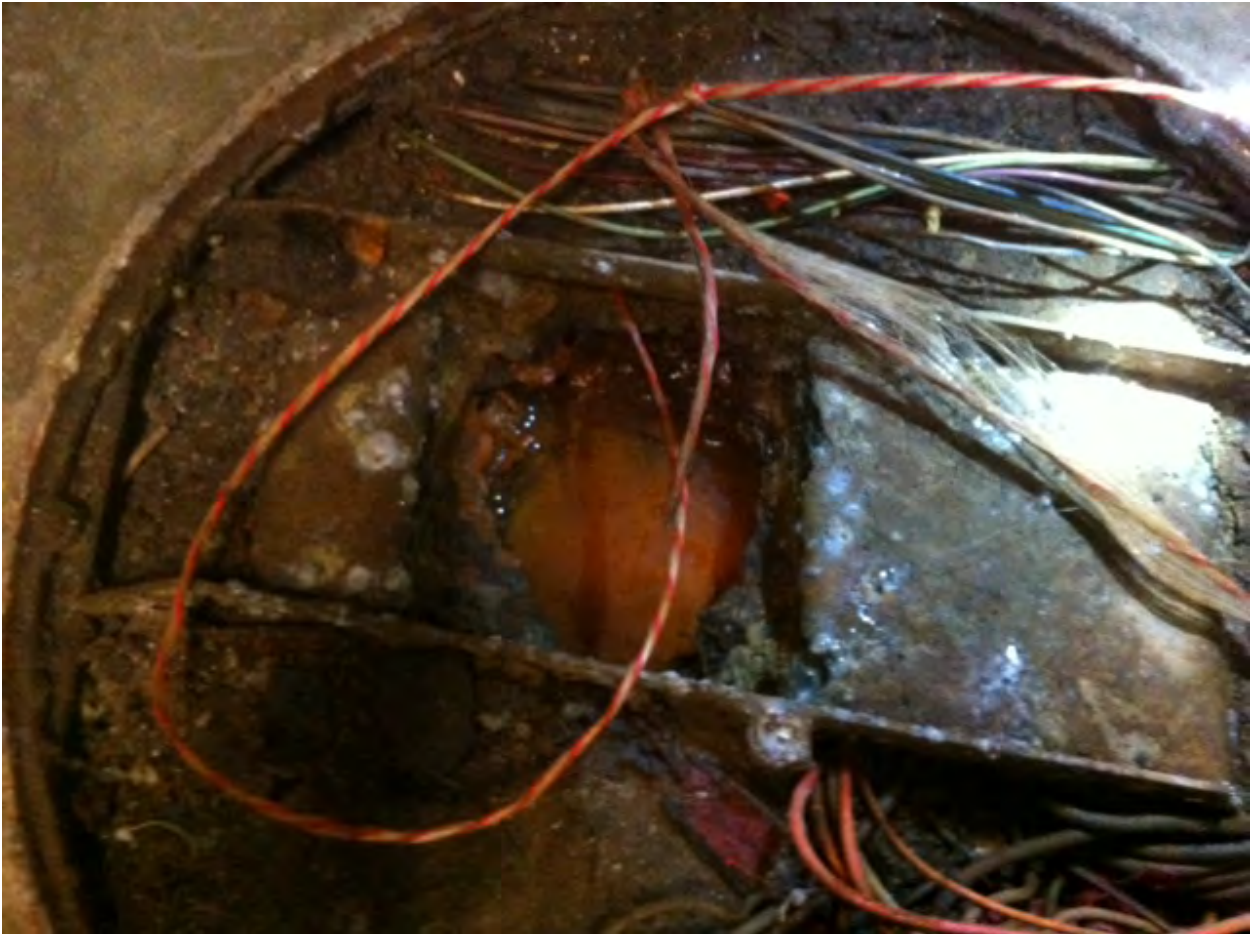
Photo 5: B07 Takoma – Standing water in first handhole
