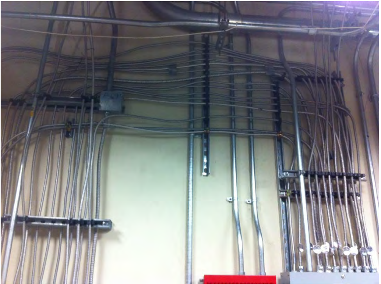
Photo #3 –Armored Flex Cables leading to AFC Panel (Electrical Room 110)
