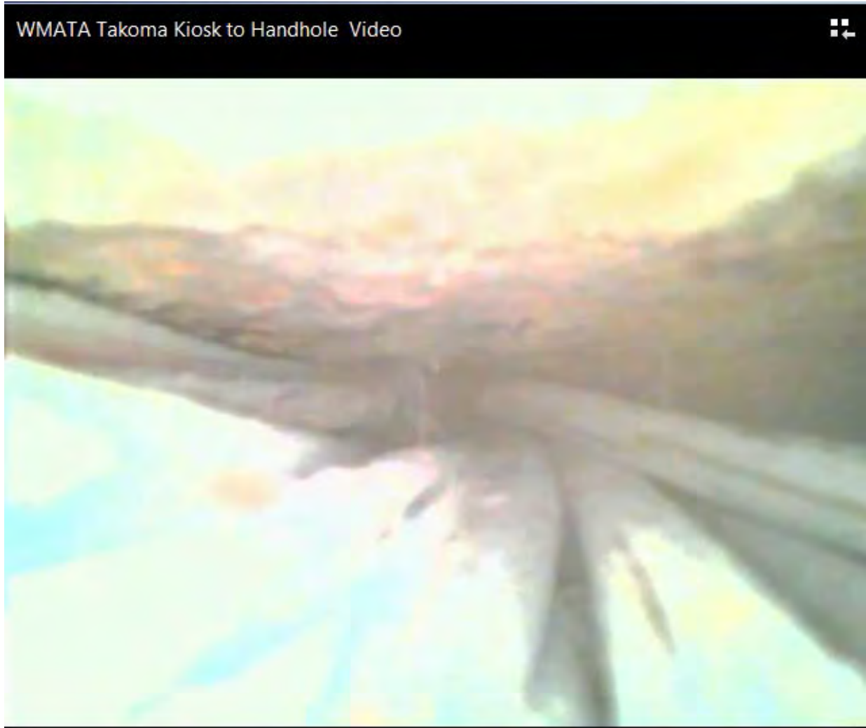
Photo #3: B07 Takoma - Still image of obstruction in power duct from kiosk to handhole
