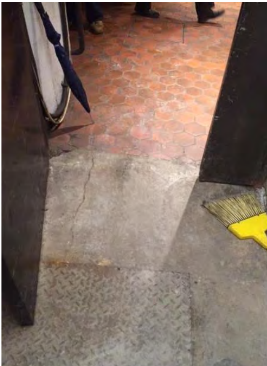
Photo #4: Entrance to backrooms and shared raceway
