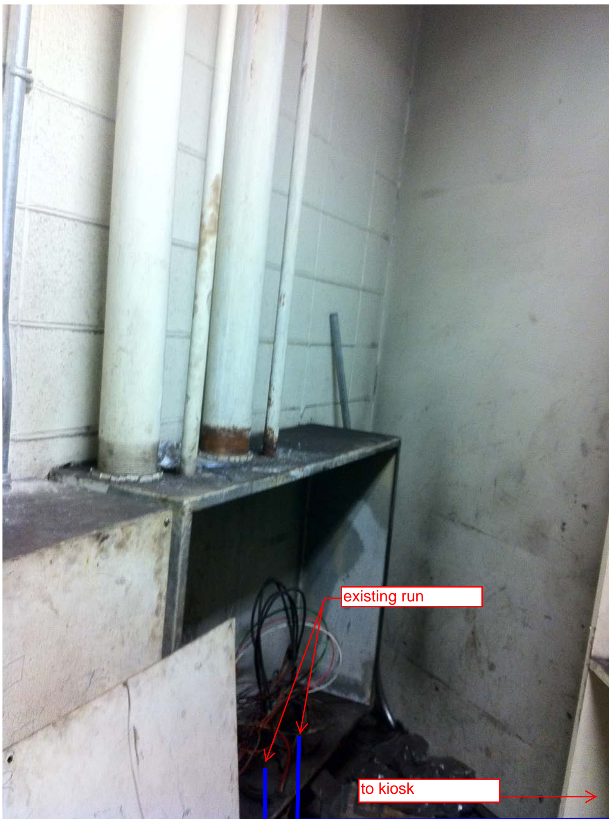
Photo #1 – A03 Dupont Circle South: Shared pull box in Verizon room #203
