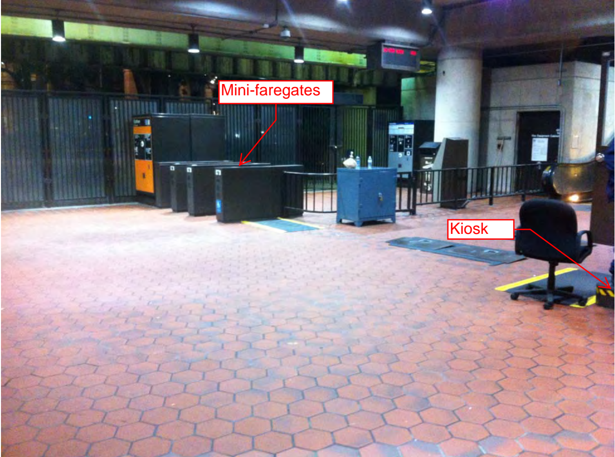
Photo #3 – Mini-faregates on mezzanine floor
