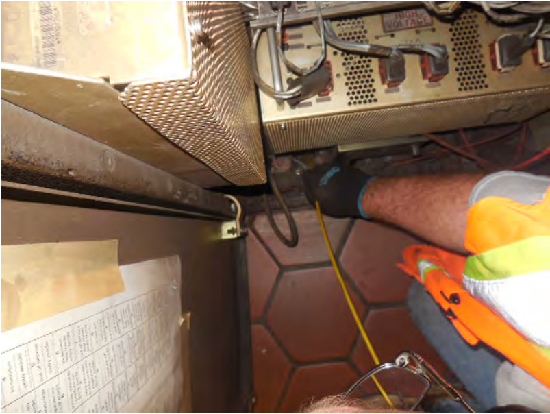
Photo #5: B10 Wheaton: Attempting to rod the faregate array ducts
