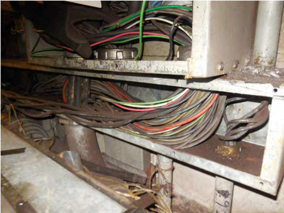
Photo #7: A08 Friendship Heights – Cable trough below AFC Panel. Power ducts from kiosk feed into bottom of trough
