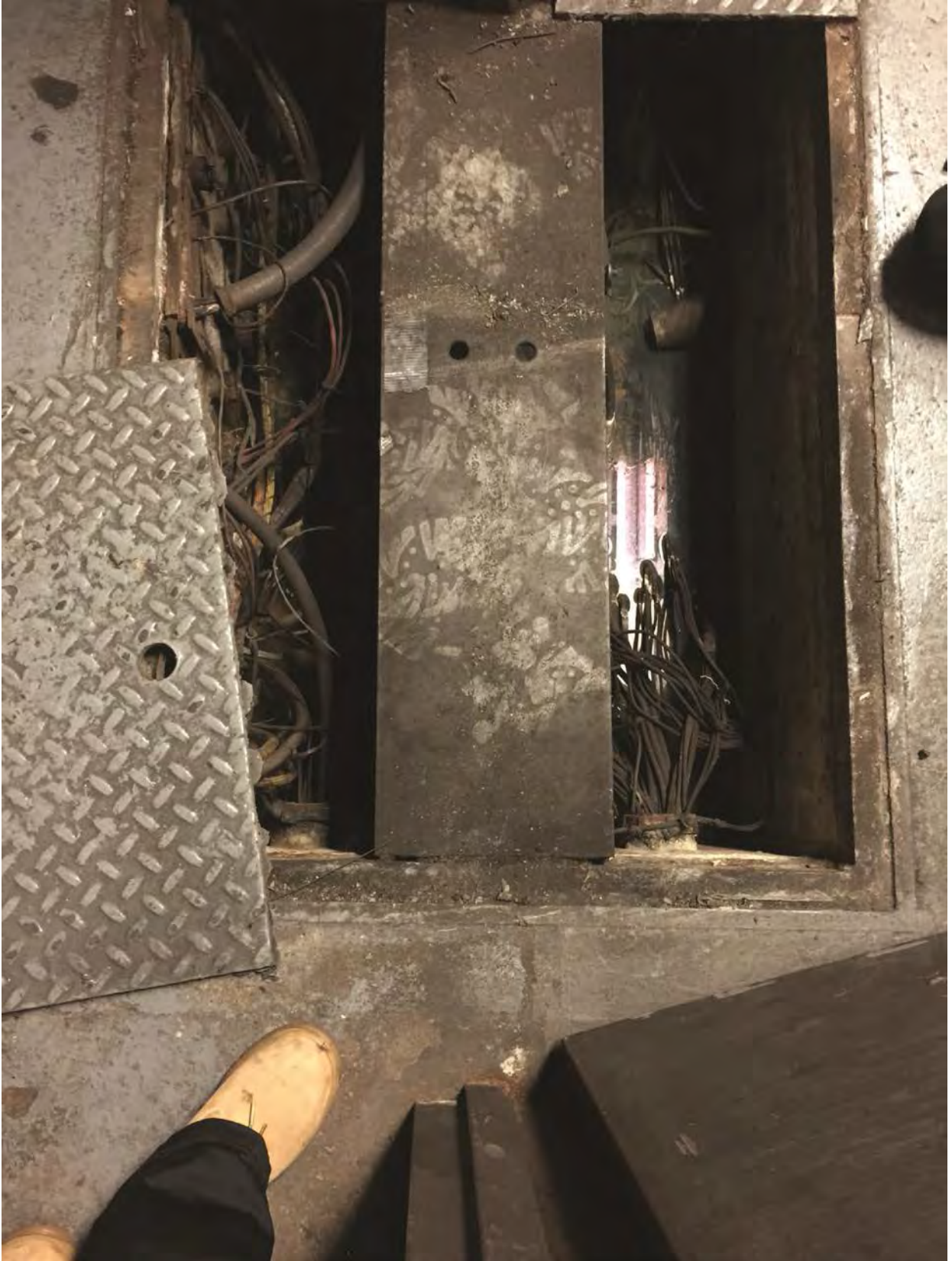
Photo #3 – A04 Woodley Park: Standing water in electrical trough
