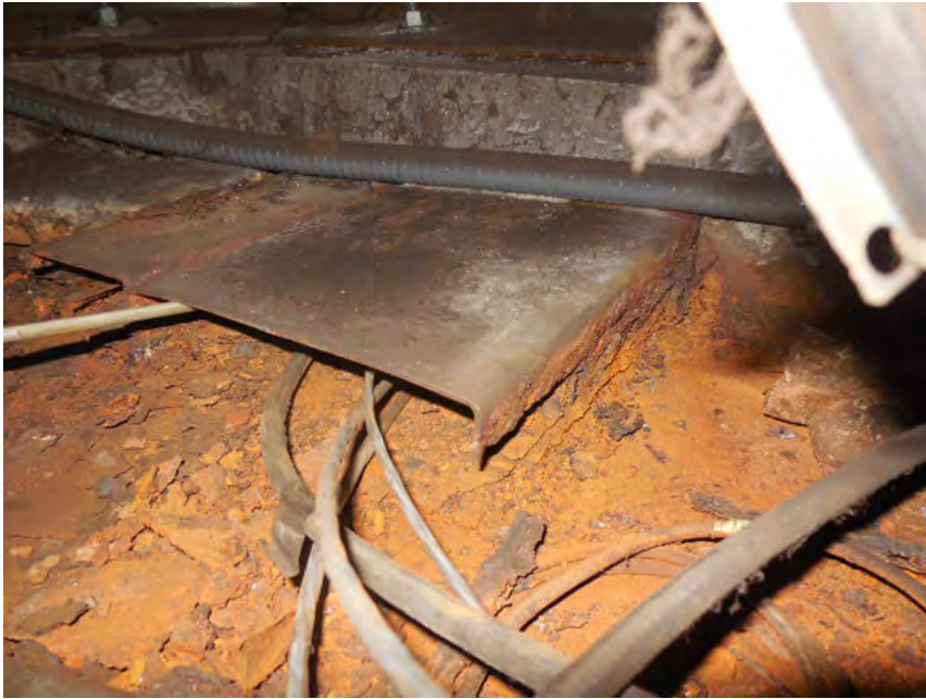
Photo #6: B10 Wheaton: Corroded communications duct opening in kiosk
