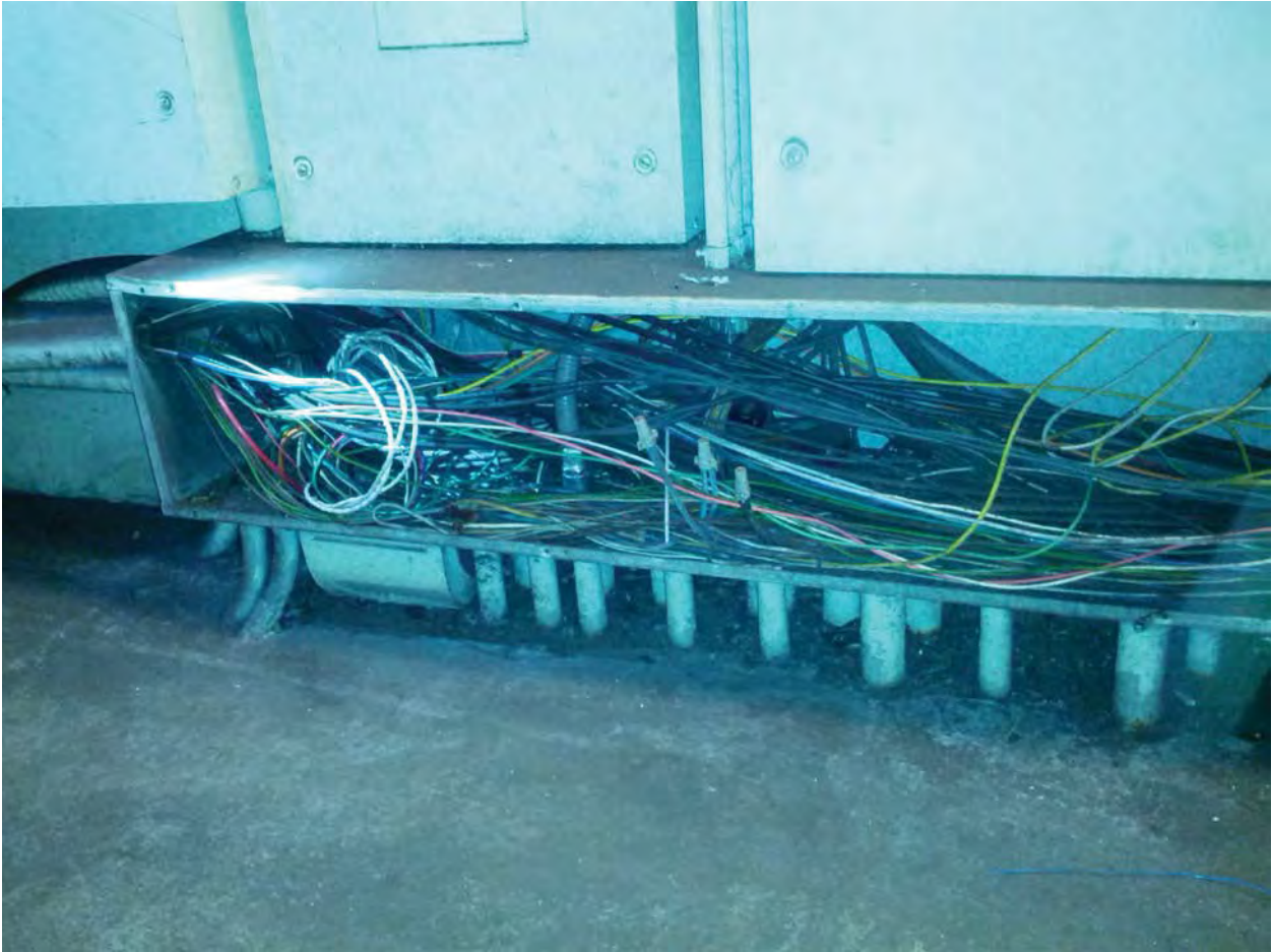
Photo #4: B02 Judiciary Square (East) – Shared cable trough in room 206. Power duct enters trough from the bottom at left.
