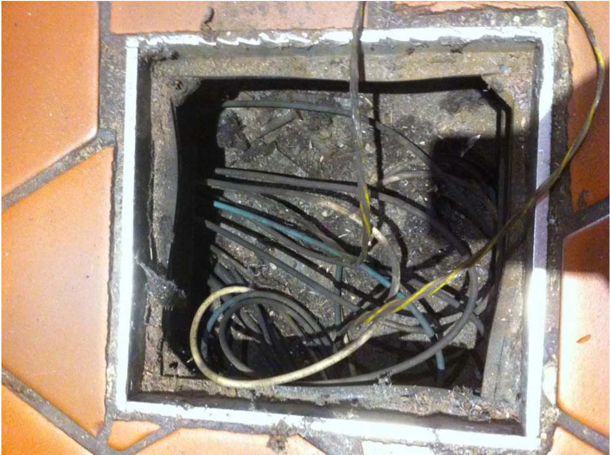
Metro Center East Photo #3 – Close-up of Hand Hole #3 to access power duct from Kiosk to AFC Panel – 12 wires counted, therefore duct is not at capacity.
