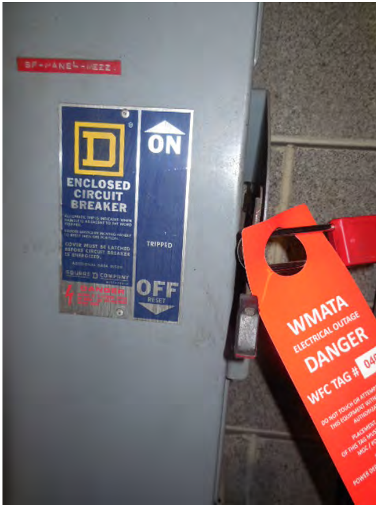
Photo #1: A12 White Flint – Lock-out tag-out of AFC Panel source breaker
