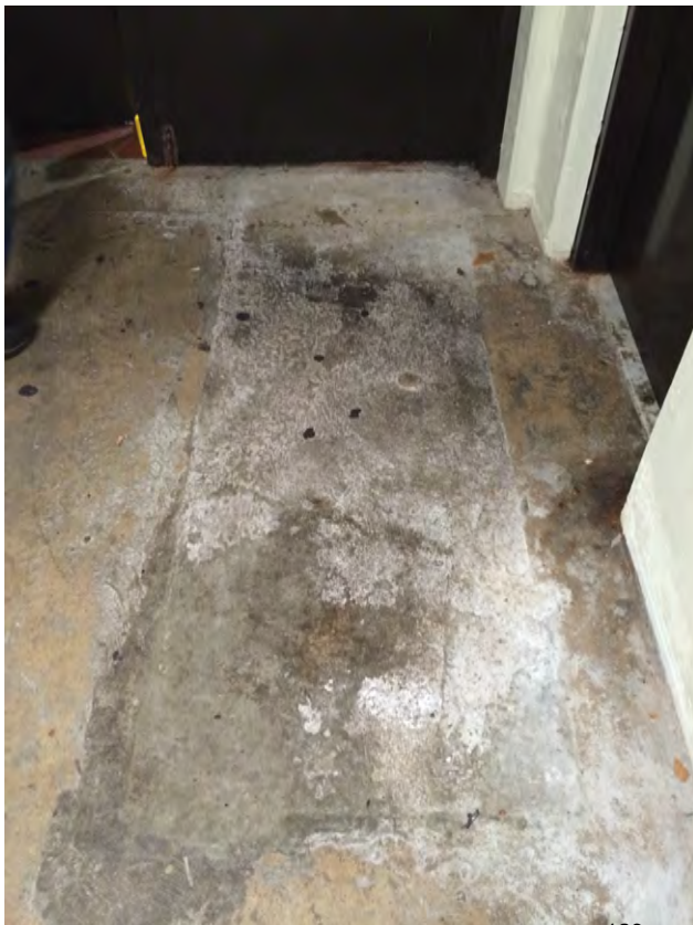
Rockville Photo #3 – Concrete repair to floor in back hallway outside Room C113
