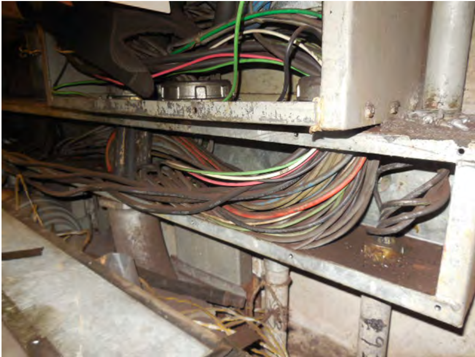
Photo #7: A08 Friendship Heights – Cable trough below AFC Panel. Power ducts from kiosk feed into bottom of trough
