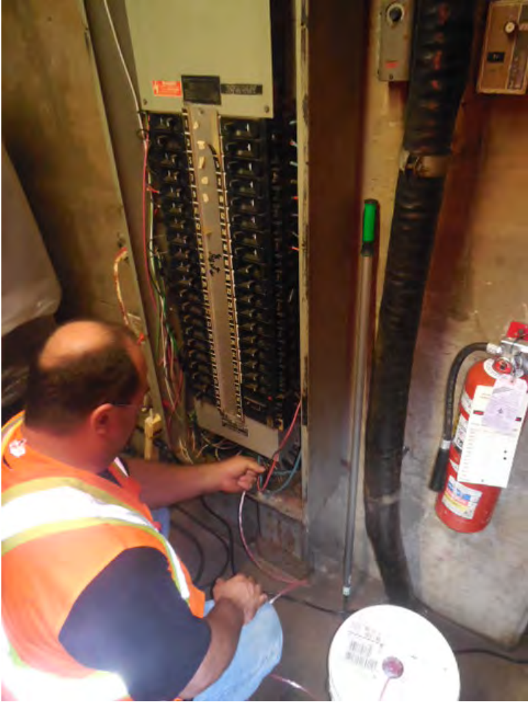
Photo #6: A12 White Flint – Pull string installation in AFC panel from kiosk
