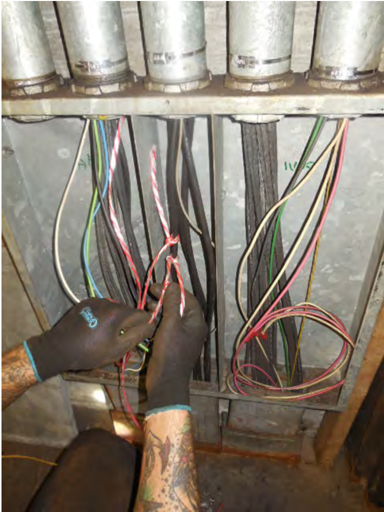
Photo #10: B10 Wheaton: Installing the pull string in the junction box near the AFC panel
