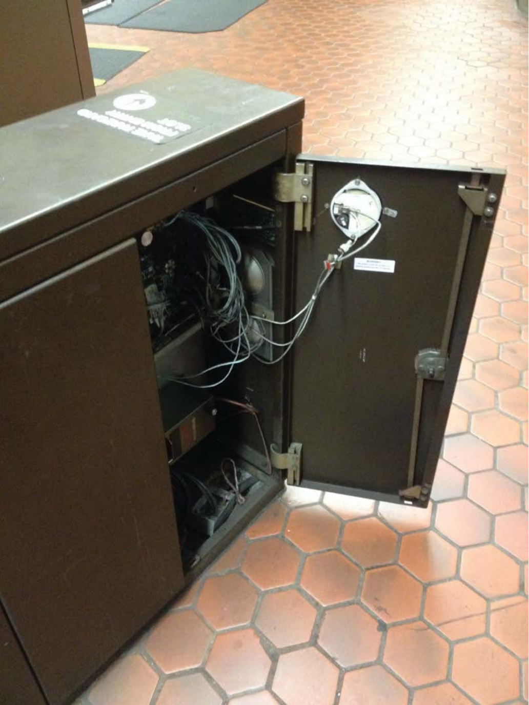
Photo #1: B02 Judiciary Square (East) – Faregate with new comm. duct and cable installed
