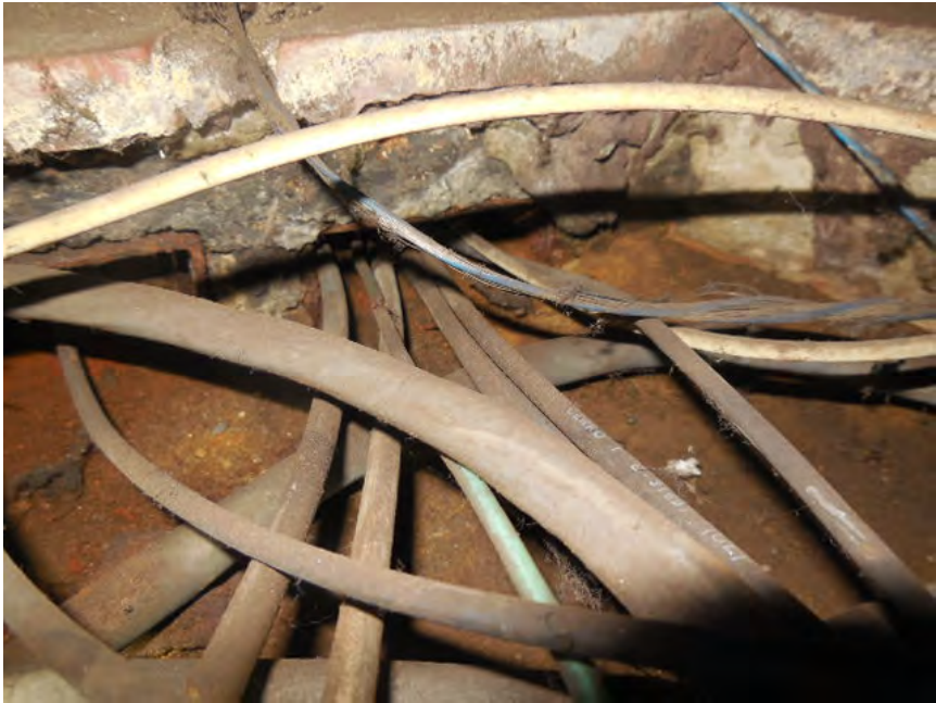
Photo #3: A12 White Flint – Power duct under kiosk floor under capacity
