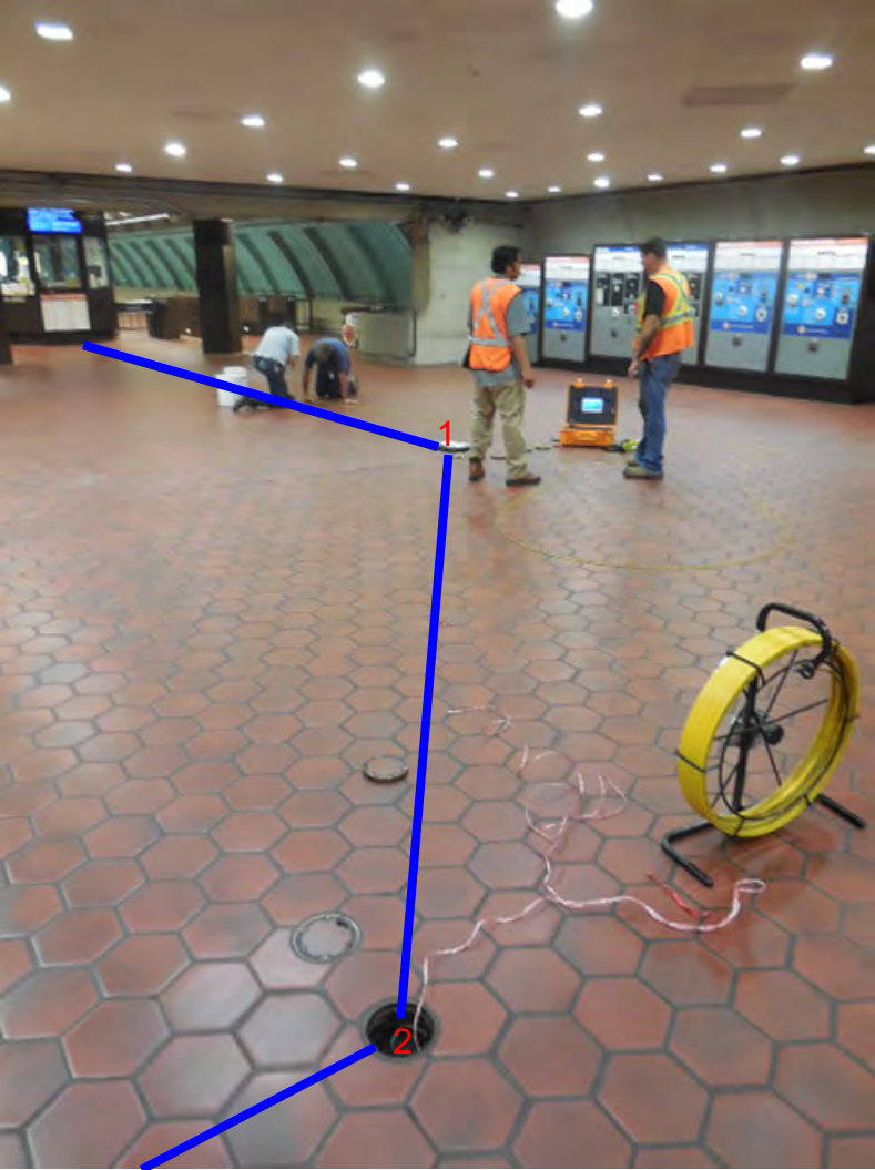
Photo #5: A08 Friendship Heights – Installing pull string in handholes between kiosk and AFC panel
