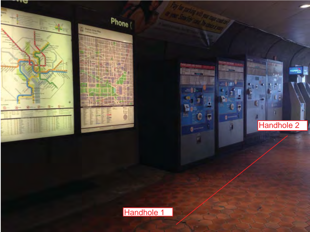
Photo #3: B02 Judiciary Square (East) – Mezzanine level handholes. Power duct run is through handholes at the bottom center and center-right of photo. Handhole near the center of photo is not part of power duct run.
