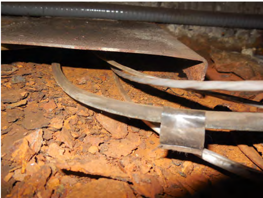
Photo #7: B10 Wheaton: Corroded communications duct opening in kiosk
