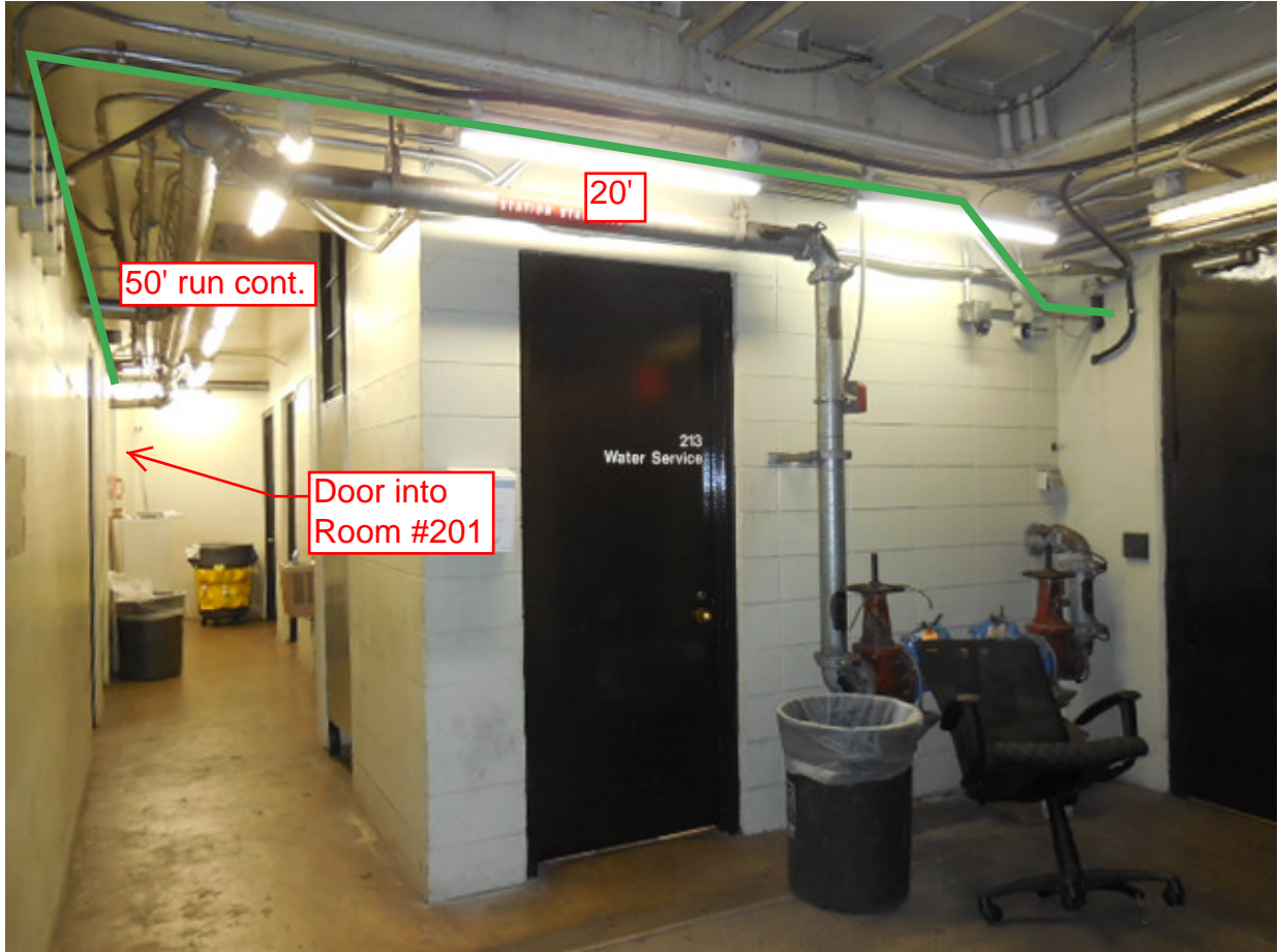
Photo #7 – A03 Dupont Circle South: Proposed conduit run continuing down hallway of room #201 and towards room #215
