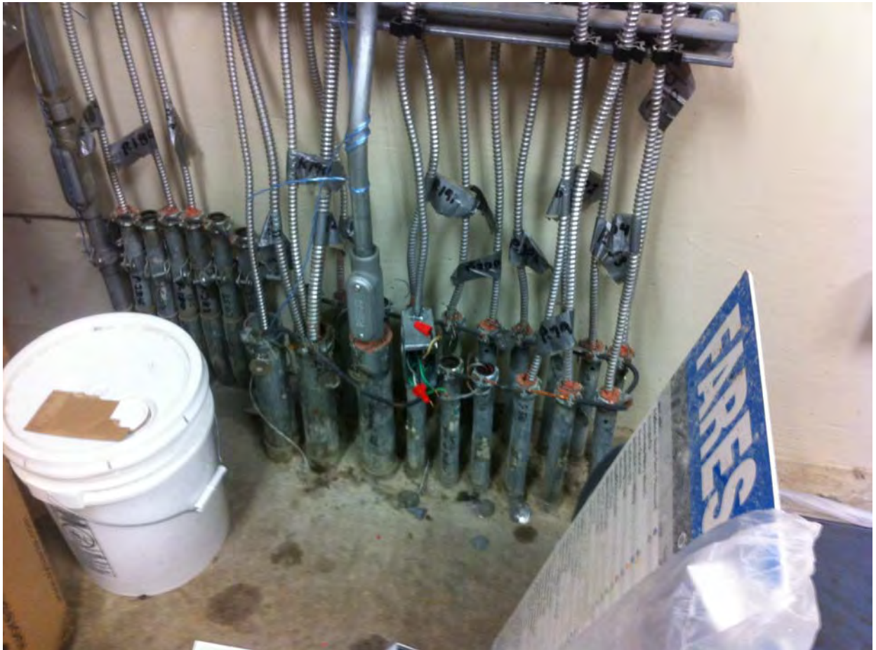
Photo #2 – Power Conduit transition to Armored Flex Cables leading to AFC Panel (Electrical Room 110)
