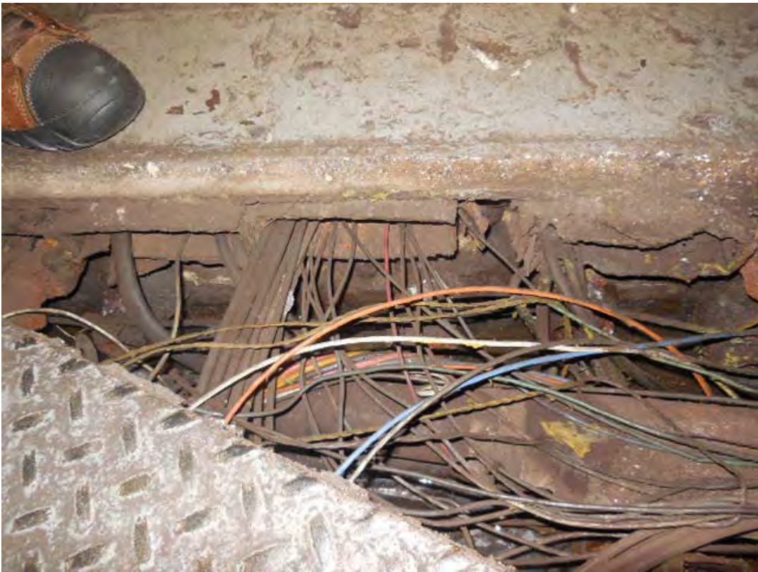
Photo #3 – Ducts from Handhole 2 entering Trench 1 in Room # 200
