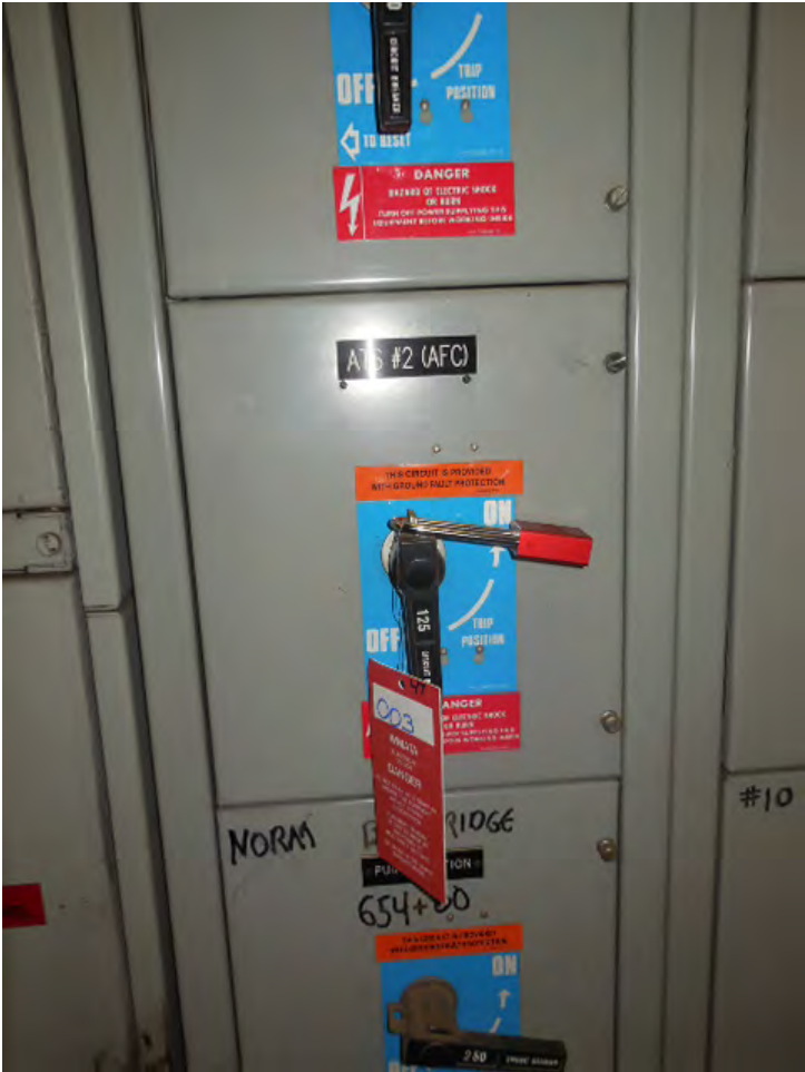
Photo #1: B10 Wheaton: Lock-out Tag-out of the feed breakers for the AFC Panel
