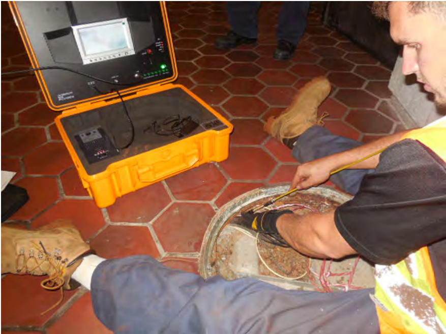
Photo #6: A13 Twinbrook – Video-scoping between kiosk and mezzanine handhole
