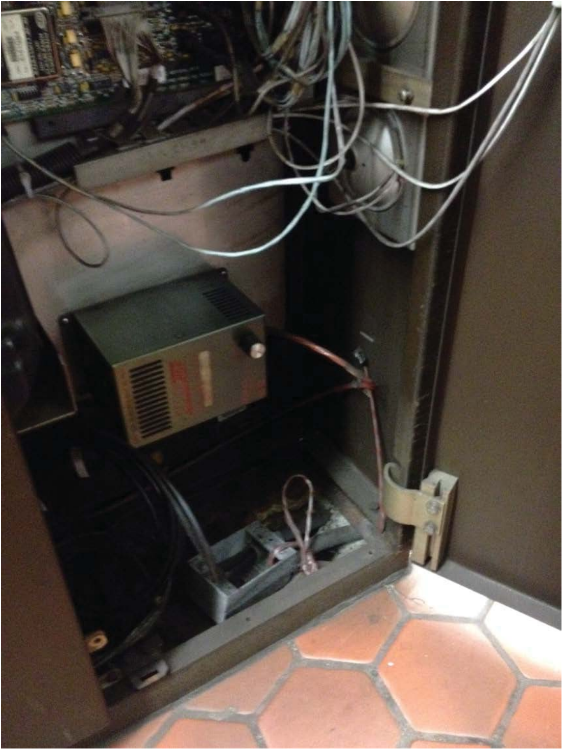
Photo #2: B02 Judiciary Square (East) – Faregate with new comm. duct and cable installed
