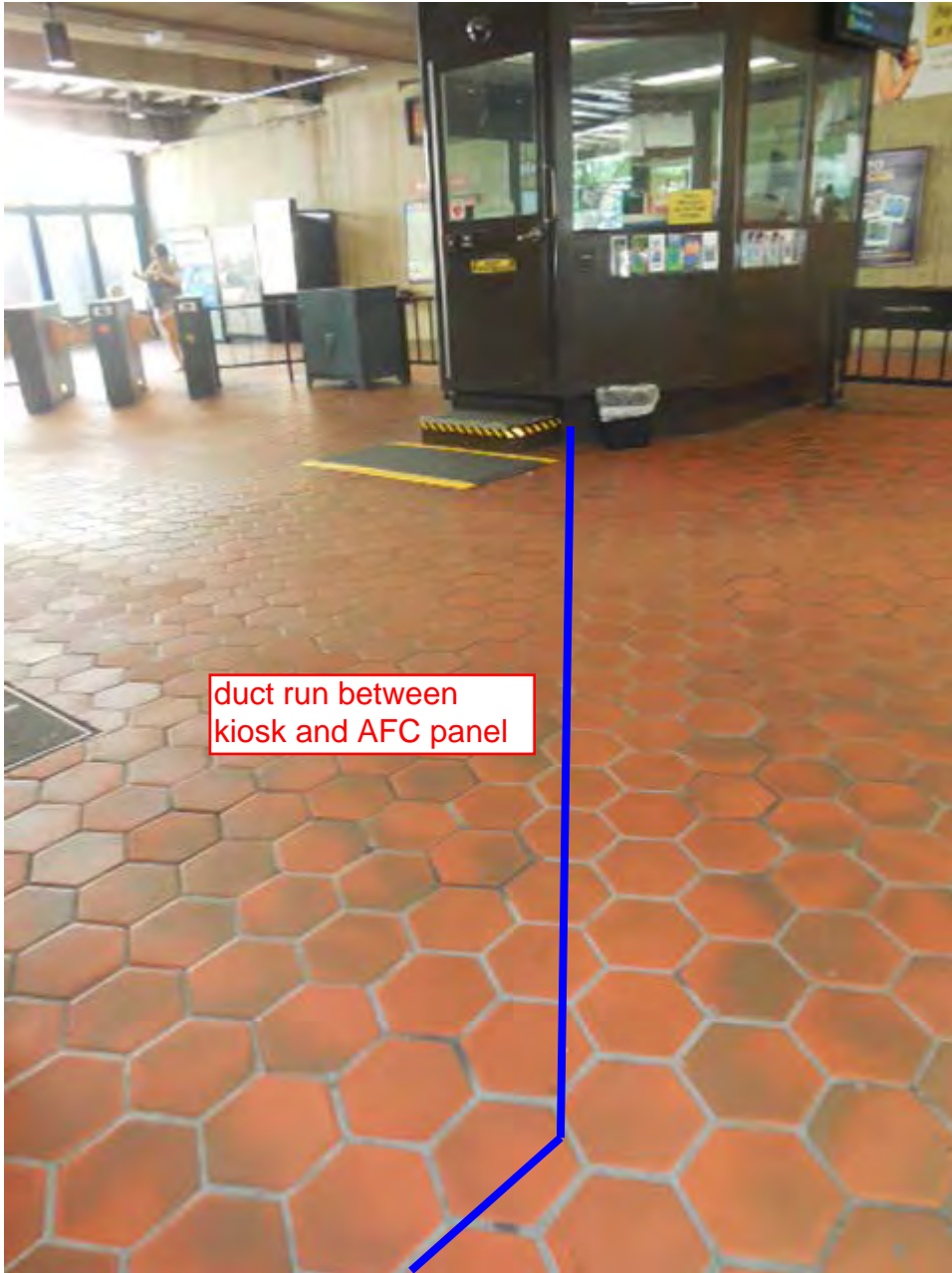
Photo #1 – B08 Silver Spring North: Kiosk on Mezzanine level
