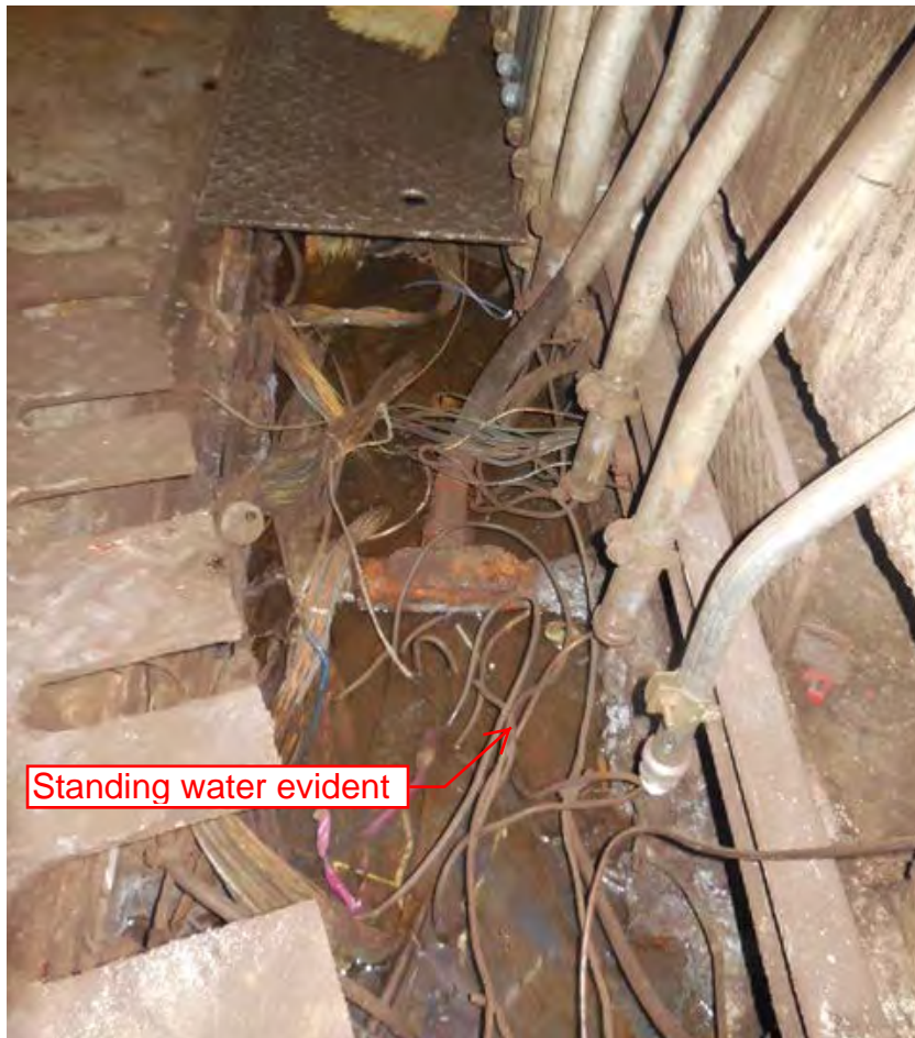
Photo #4 –Trench 1 in Room # 200 with overhead conduit transition, standing water evident.
