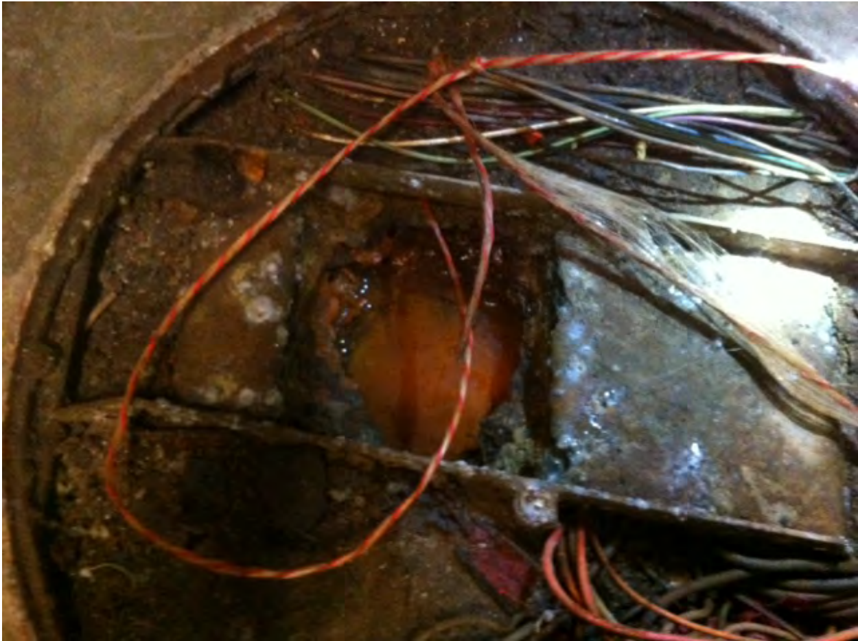
Photo 5: B07 Takoma – Standing water in first handhole
