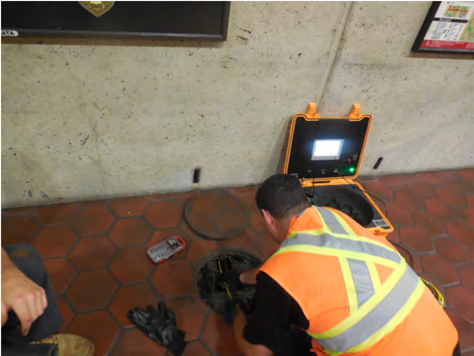
Photo #6: A08 Friendship Heights – Video-scoping the power ducts between kiosk and AFC panel
