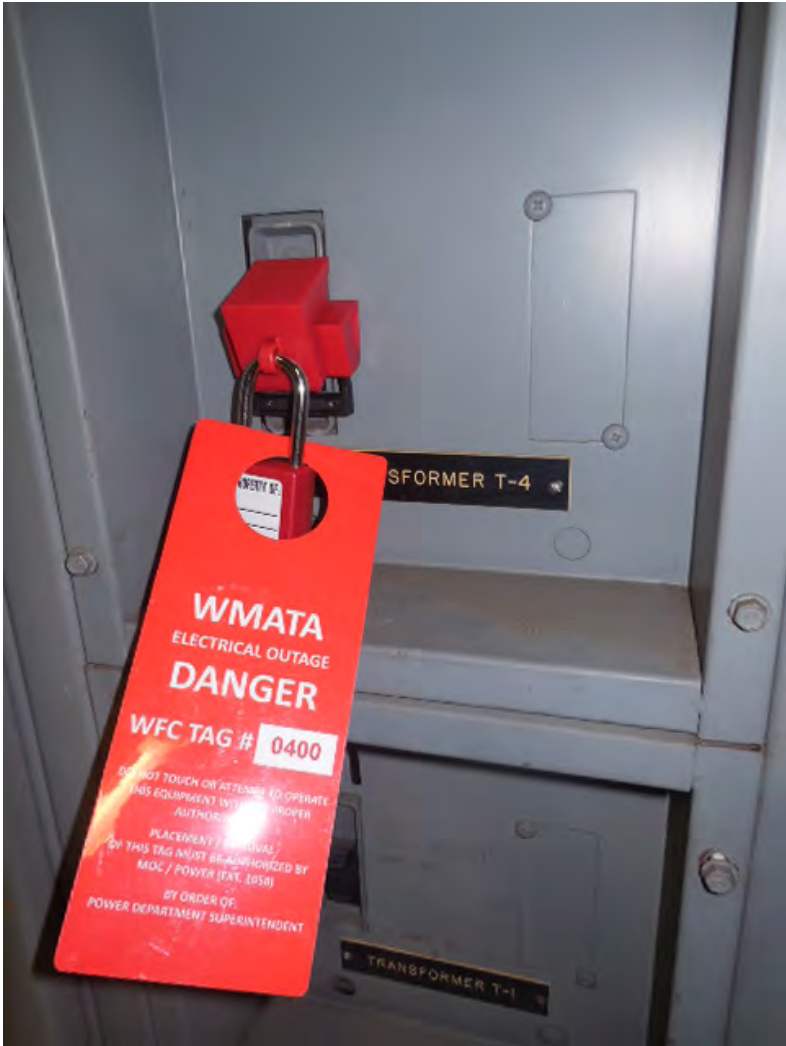
Photo #1: A13 Twinbrook – Lock-out tag-out of feeder breaker to AFC Panel
