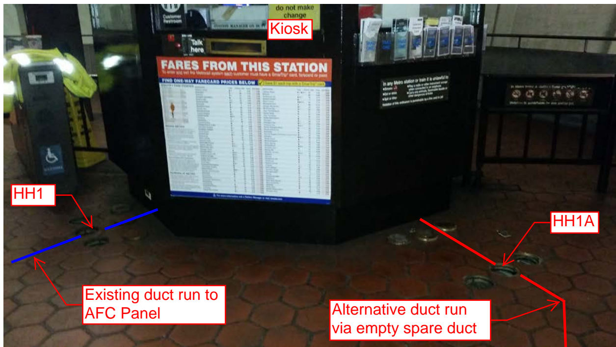
Photo #2: Existing & alternate power duct from to Kiosk to handholes.
